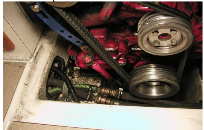
Still a Mess even after Cleaning Up and New Belts
